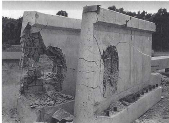
Figure 1.1: Reinforced concrete after EFP impact.(2)
